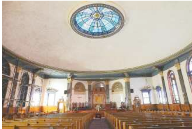
The beautiful sanctuary at the Free Synagogue of Flushing needs restoration. Some windows have already been removed and leaks threaten the stained-glass dome. PHOTO BY PJ SMITH
